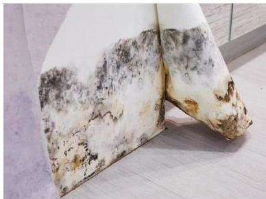
Mold and Fungus
